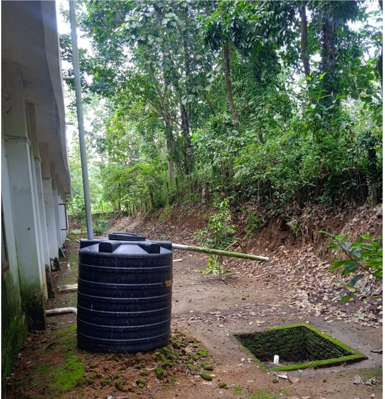
Rain Water Harvesting Unit
